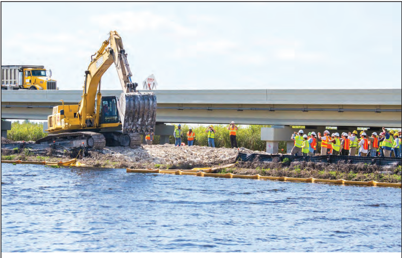
Following the completion of the 1-mile bridge along the Tamiami Trail, crews commenced removal of the existing roadway in May of 2012. NPS photo.
